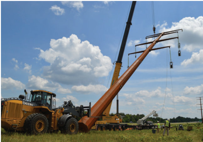
The overall Hampton-Rochester-La Crosse transmission project was completed in 2016. (Photo courtesy of CapX2020.)
